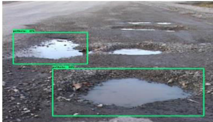
Fig.3. Pothole Output Detection
